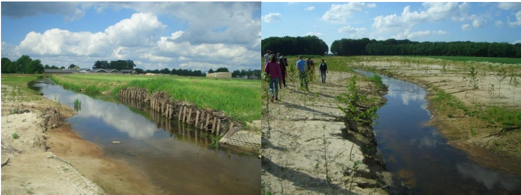
Figure 15 Remeandering, lowering of the surrounding floodplain, shoreline protection with wood and tree planting (so-called 2-stage profile)
